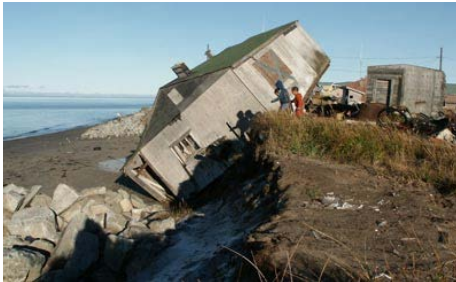
Shishmaref home lost to erosion alaskaconservation.org , accessed January 19, 2013
